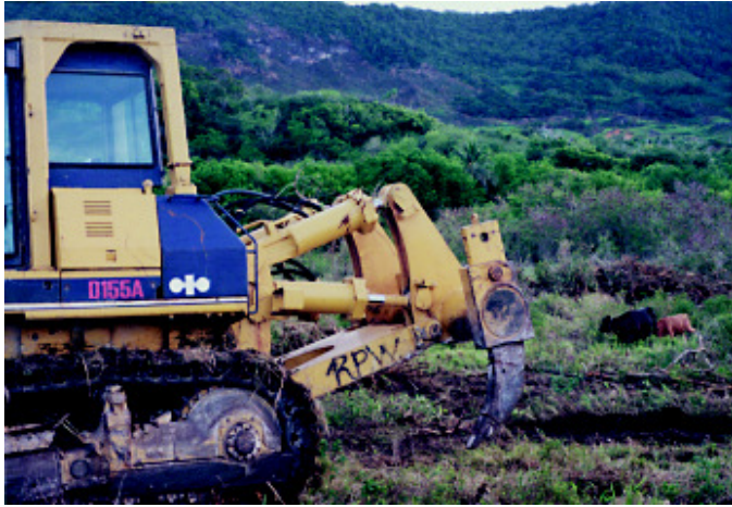
Development such as earthmoving that reduces an endangered species' critical habitat requires a federal permit.
